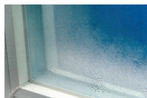
Metal Window Spacer may cause condensation and toxic mold
